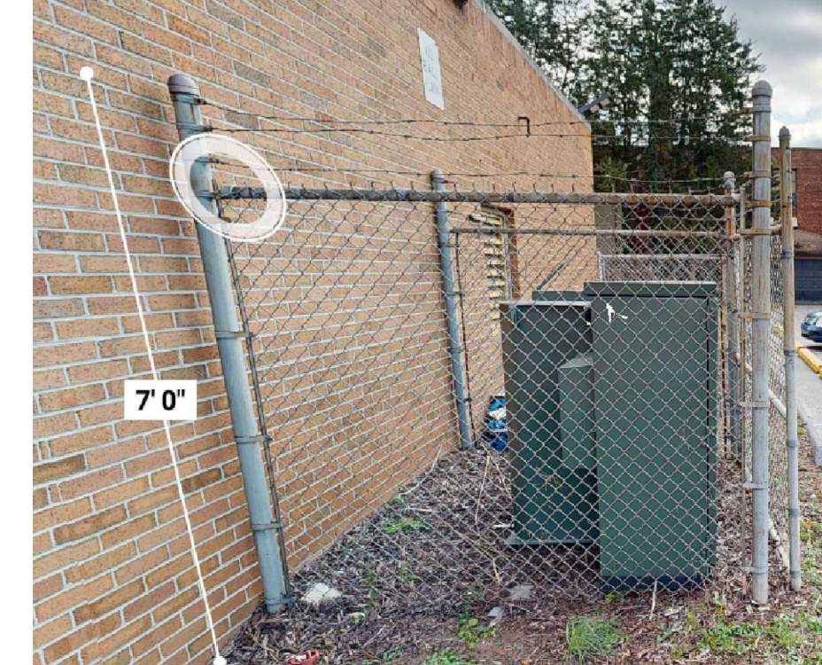
EXISTING 7 FT HIGH CHAIN LINK TRANSFORMER ENCLOSURE
